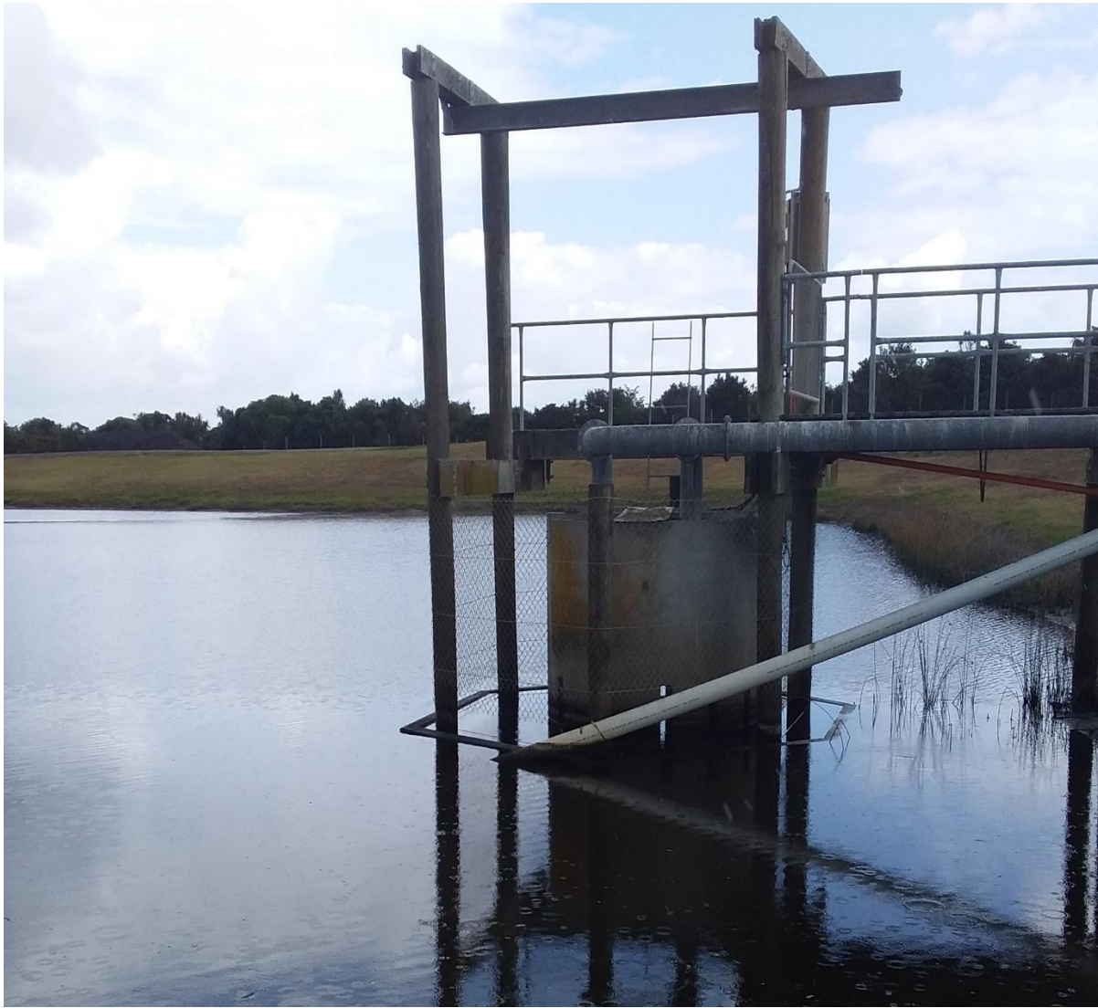
Figure 8 - Discharge Well with the two discharge pumps inside and effluent measuring
